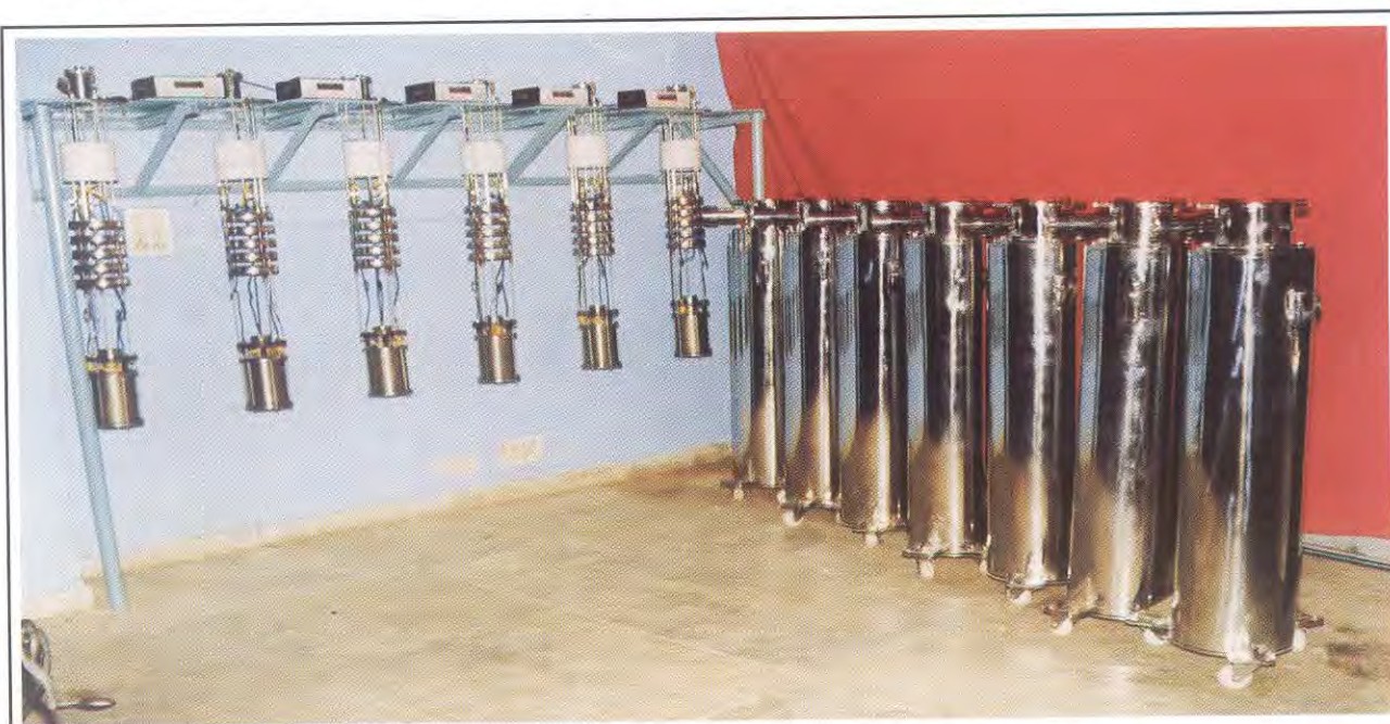
Fig.8.1 : The six 7 Tesla SC Magnets (50 mm. bore dia.) with suspension system. LHe level meters and seven nos. of bucket type LHe cryostats.
