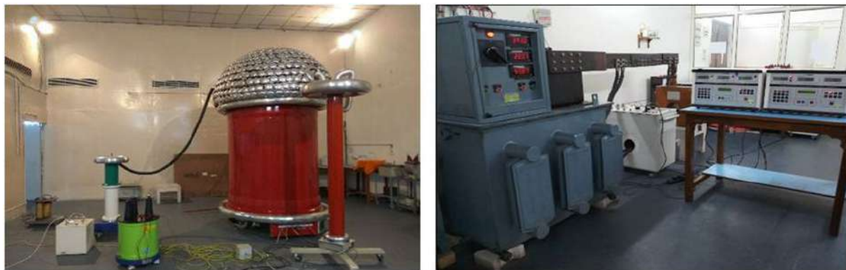
Measurement set-up for AC High Voltage (left) and AC High Current (right)
